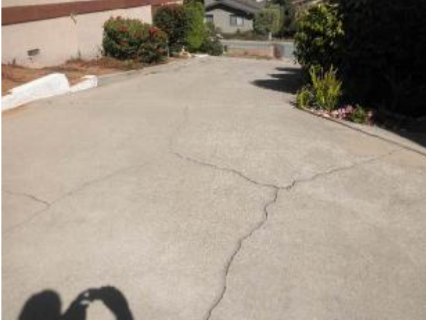
General settlement cracks in the concrete driveway.
