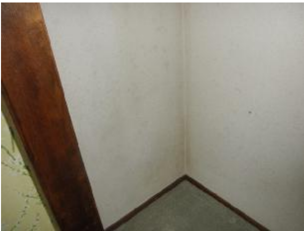
Brown mildew like substance on the drywall inside the closet.
