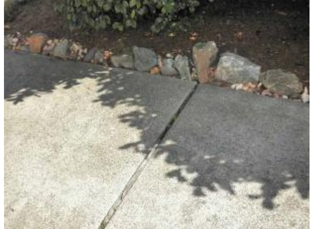
Damaged and missing wood spacers in the concrete driveway.
