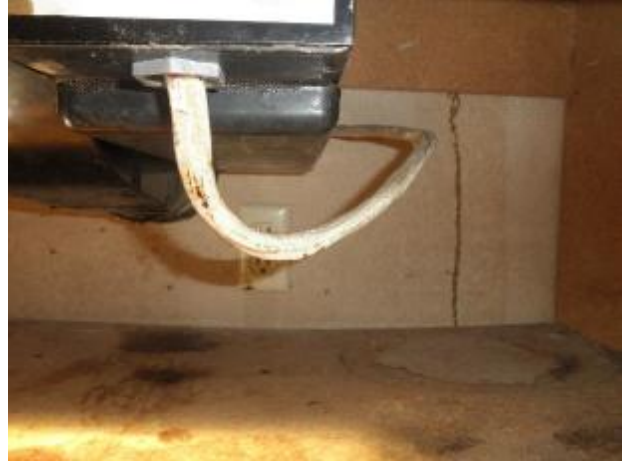
Missing conduit at the Romex wiring in the cabinet below the kitchen range.
