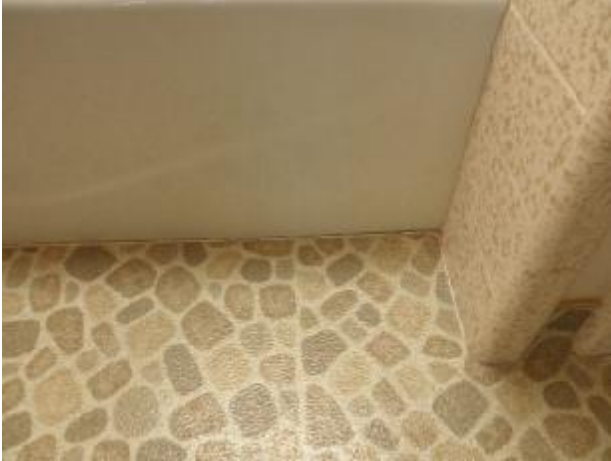
Seal gaps where the vinyl flooring interfaces with the tub and shower in the master bathroom.
