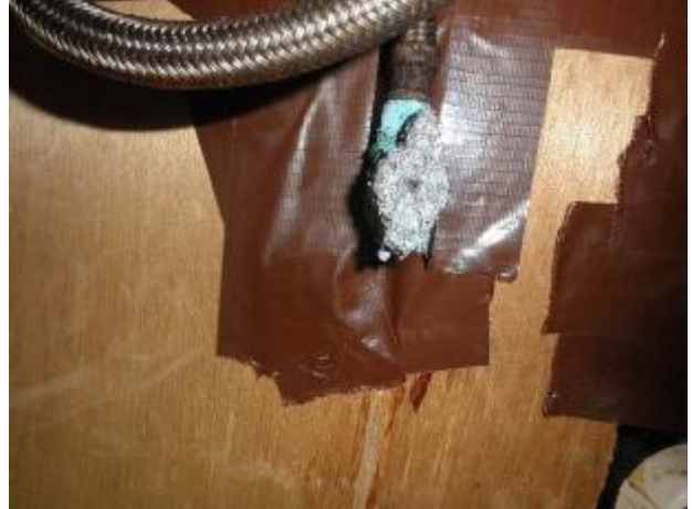
Excessive corrosion on the angle stop valves below the sink in the hall bathroom.
