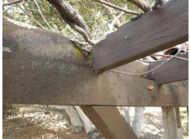
Moisture damage to the framing at the pergola.
