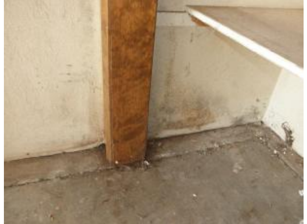
Evidence of leaks with a black mildew like substance on the drywall inside the garage.
