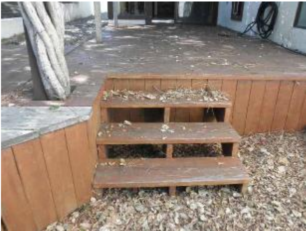
Missing railing at the backyard deck stairs.
