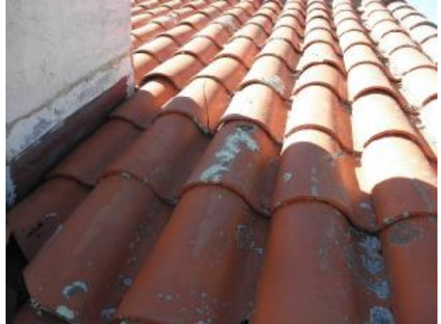
Example of the cracked and broken roof tiles.
