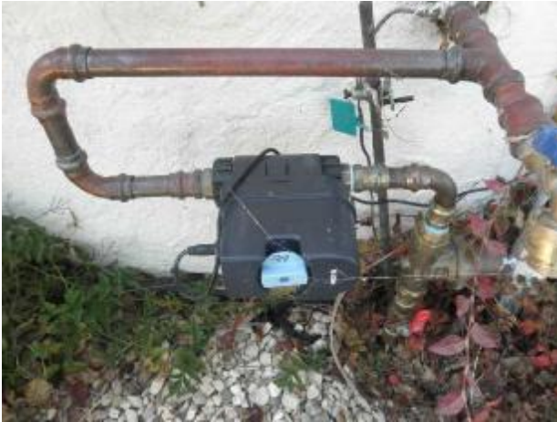
Flow sensor installed at the main water riser.
