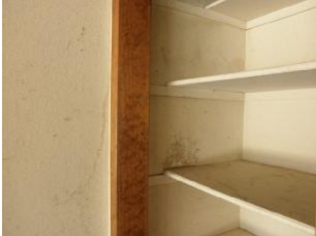
Evidence of leaks with a black mildew like substance on the drywall inside the garage.
