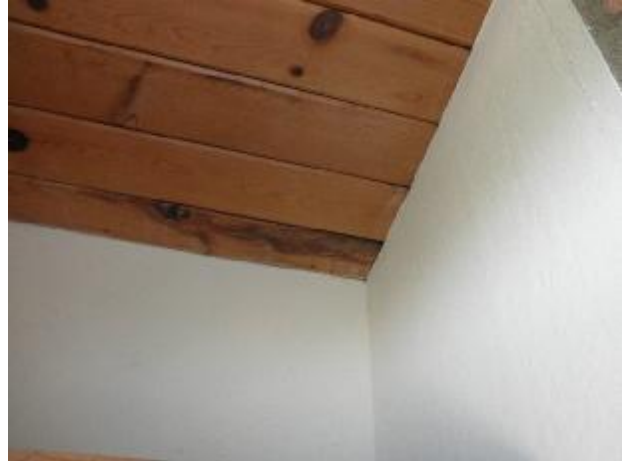
Evidence of leaks in the living room.
