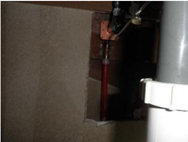
Hole in the drywall below the sink in the master bathroom.
