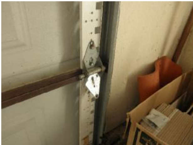
Loose roller hinge at the garage door.
