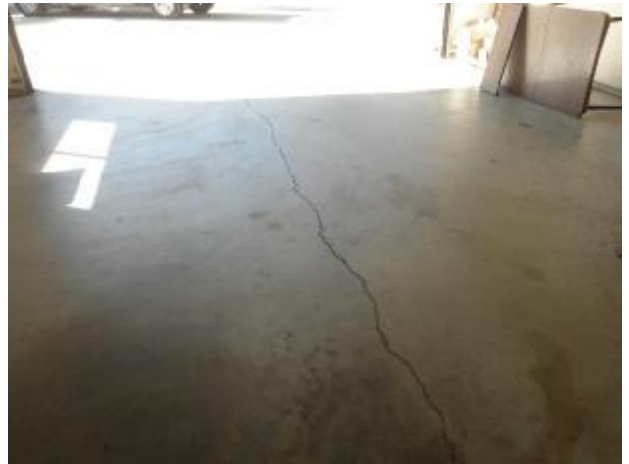
General settlement crack in the garage concrete slab.
