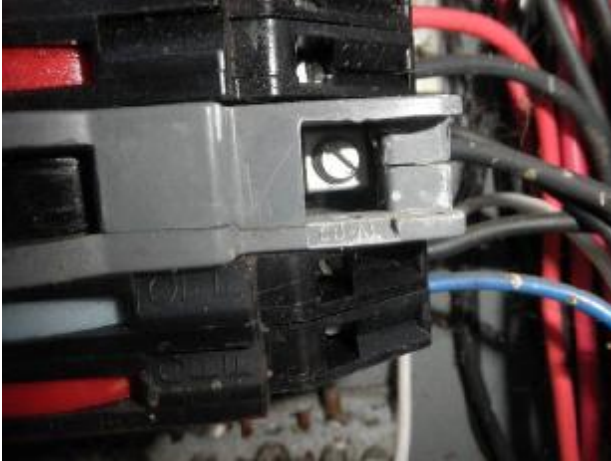
Double tapping at one of the circuit breakers in the main electrical service panel.
