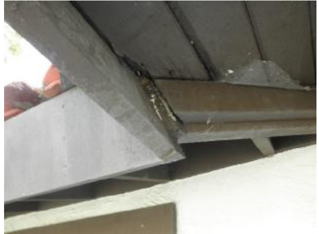
Example of the moisture and termite infestation/damage at the exterior eaves.
