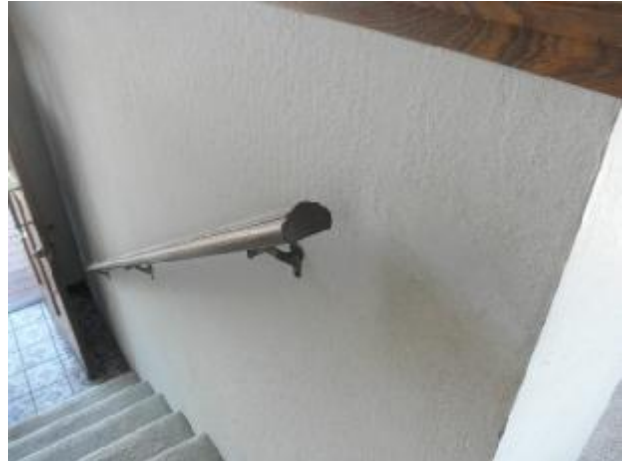
The stair railings do not return to the wall.
