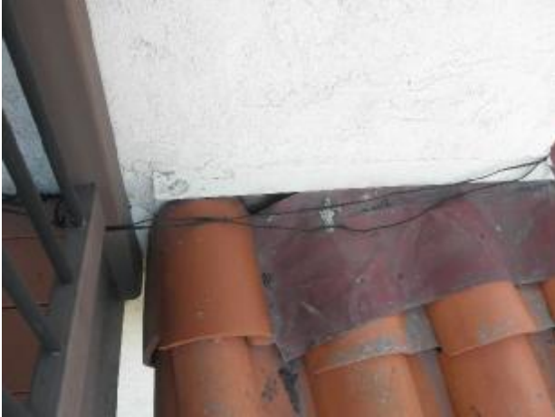
Dislodged roof-to-wall flashing.
