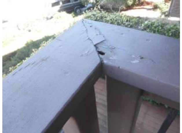
Example of the moisture and termite damage at the site decks.
