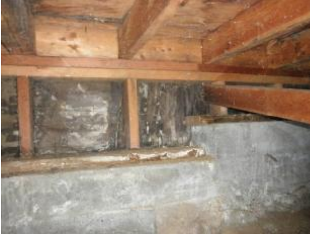
Fungus damage at the cripple wall and plywood subflooring in the substructure area.
