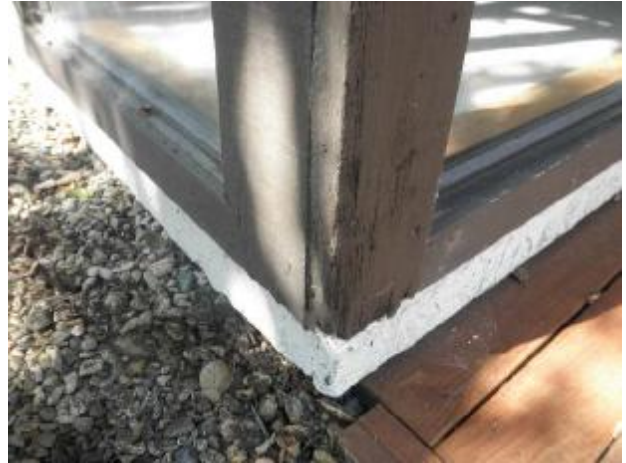
Moisture damage at the base of the exterior walls in the sun room.
