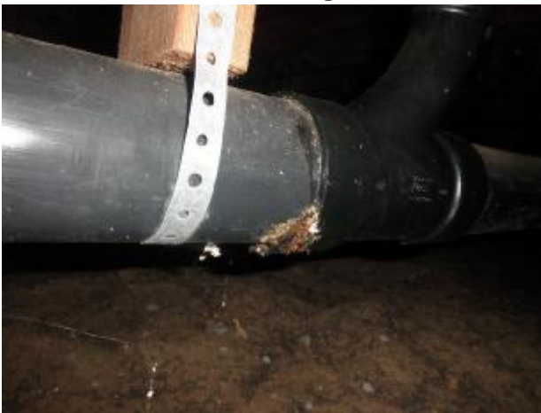
Leak at the drain waste line in the substructure area.
