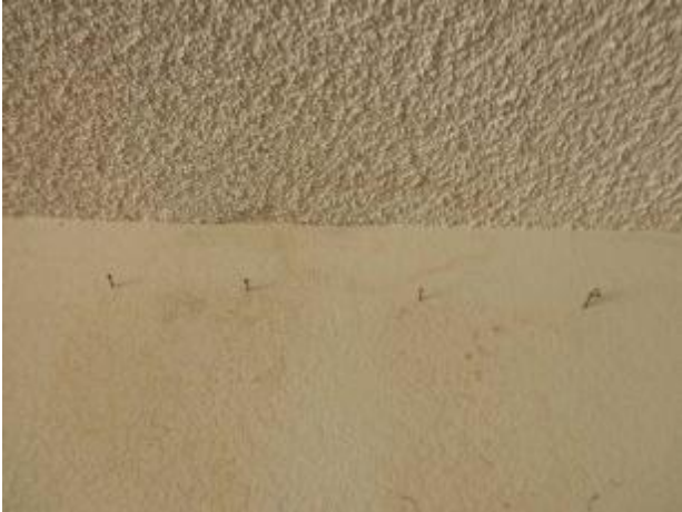
Evidence of leaks in the garage.
