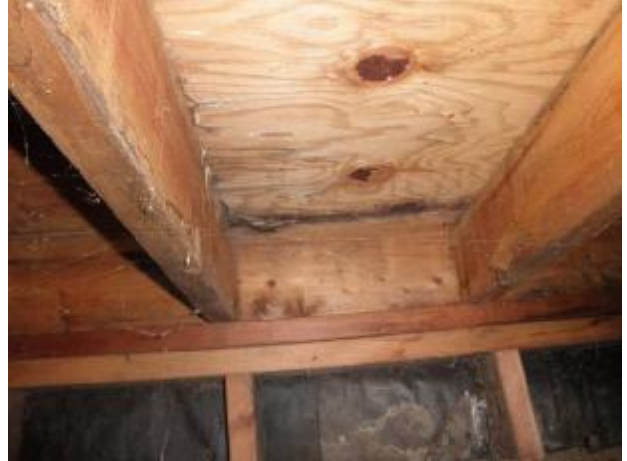
Fungus damage at the cripple wall and plywood subflooring in the substructure area.
