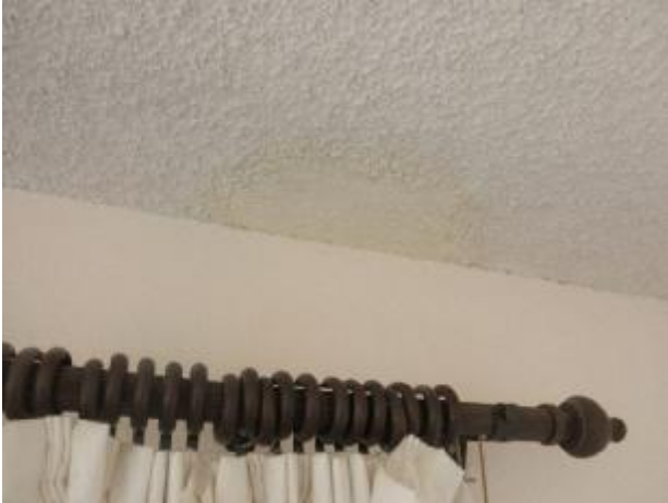
Evidence of leaks in the master bedroom.
