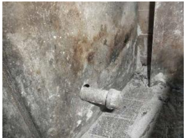
Gaps around the gas pipe in the fireplace need to be sealed.
