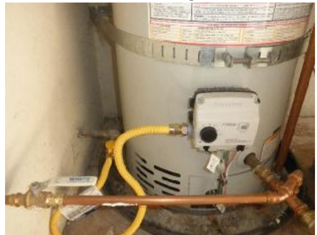
Missing sediment trap at the gas line connection to the water heater.
