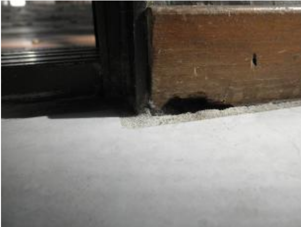
Evidence of subterranean termite infestation at the base of the sun room wall.
