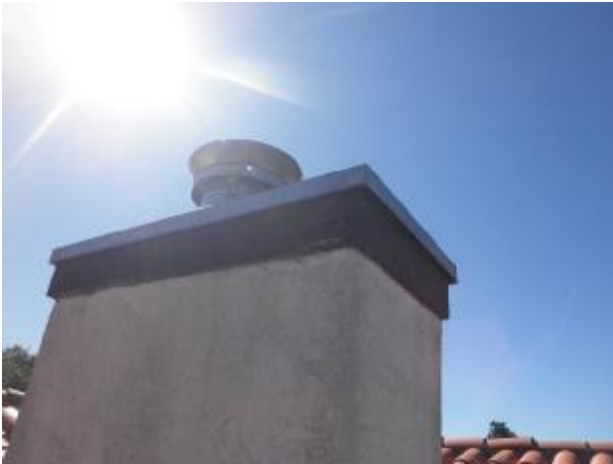
Moisture and termite damage to the wood trim at the top of the chimney enclosure.
