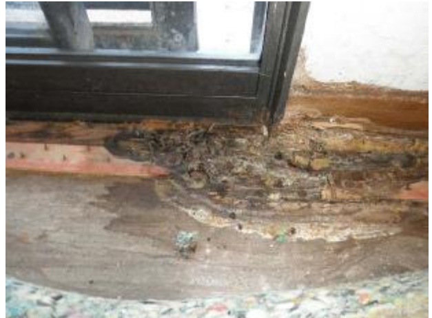
Leaks with moisture and bug damage to the interior subflooring by the sliding glass door in the dining rm.
