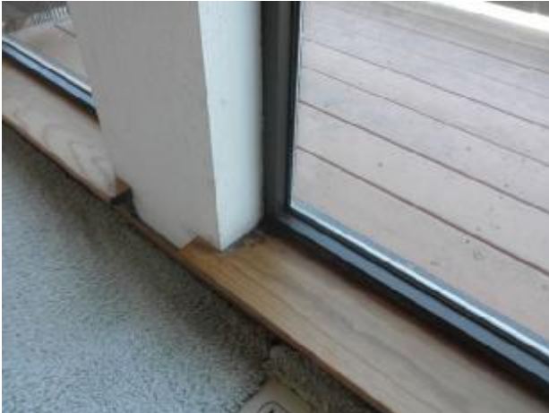
Evidence of leaks at the large fixed windows in the living room.
