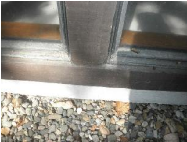
Moisture damage at the base of the exterior walls in the sun room.
