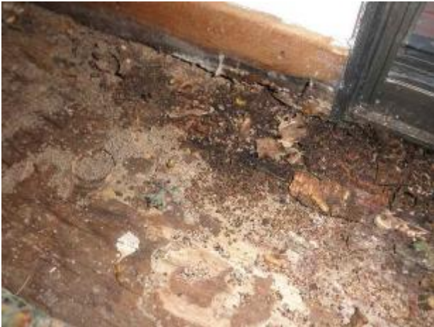
Leaks with moisture and bug damage to the interior subflooring by the sliding glass door in the mas. bed
