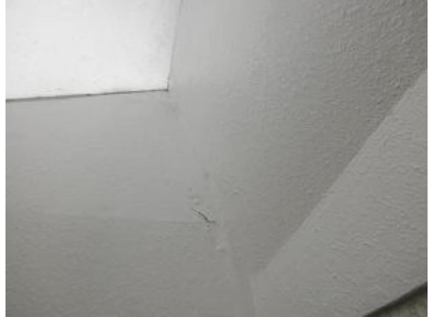
Evidence of leaks at the skylight.
